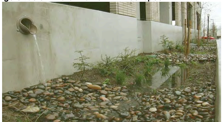
Figure 7: Stormwater Planter with Roof Spout
