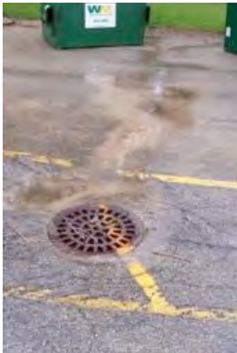
Figure 2: Rain water runoff
