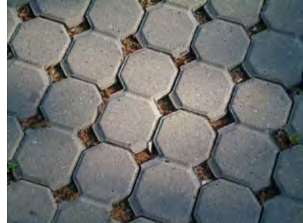
Figure 6: An Example of Porous Paving
